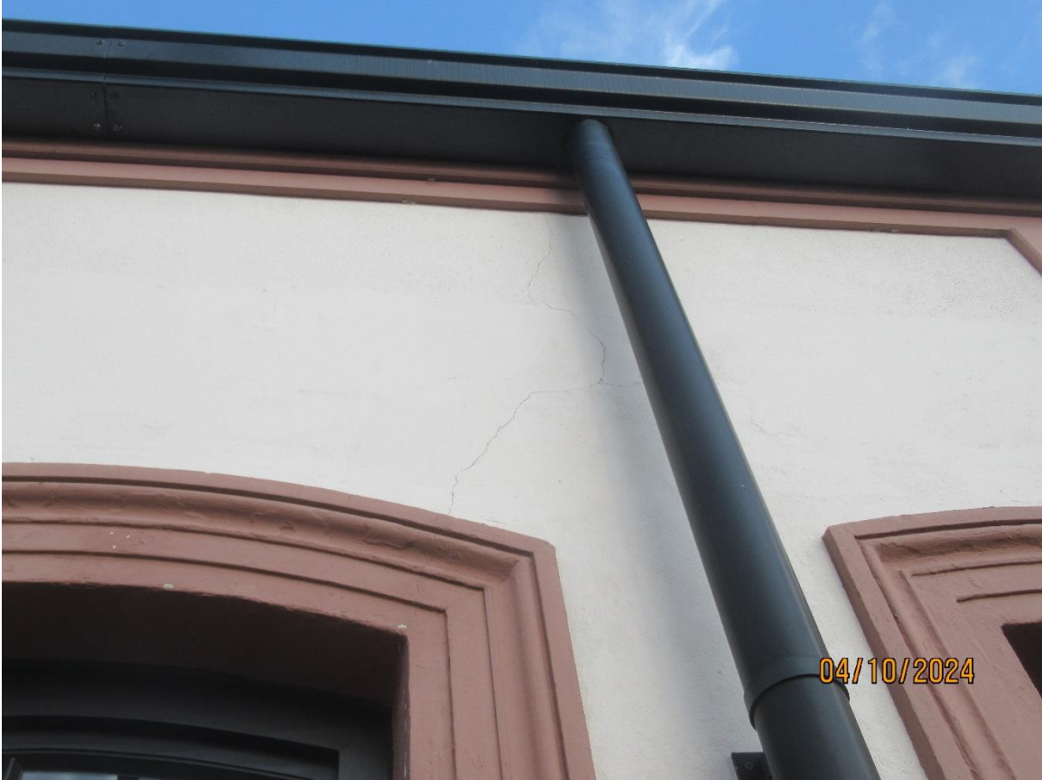
P19 – typical crack in building
