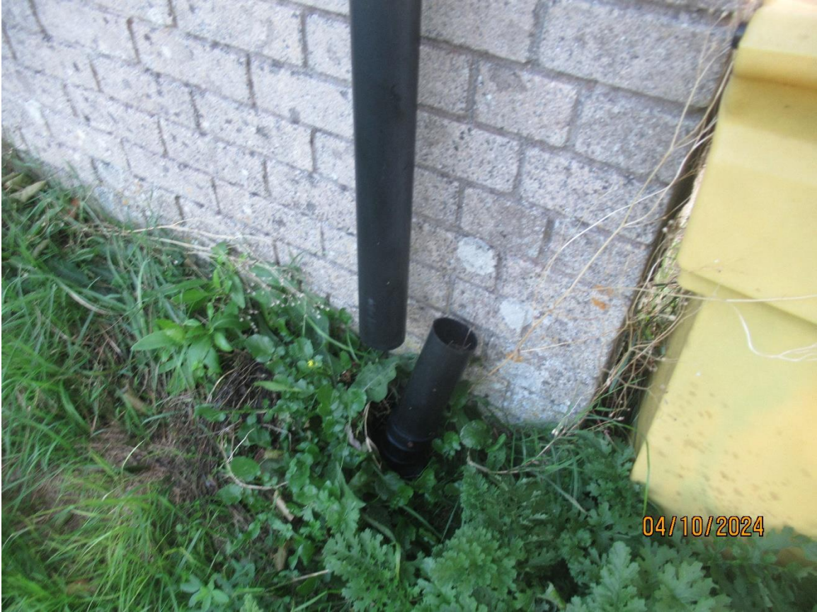
P11 – broken drainpipe
